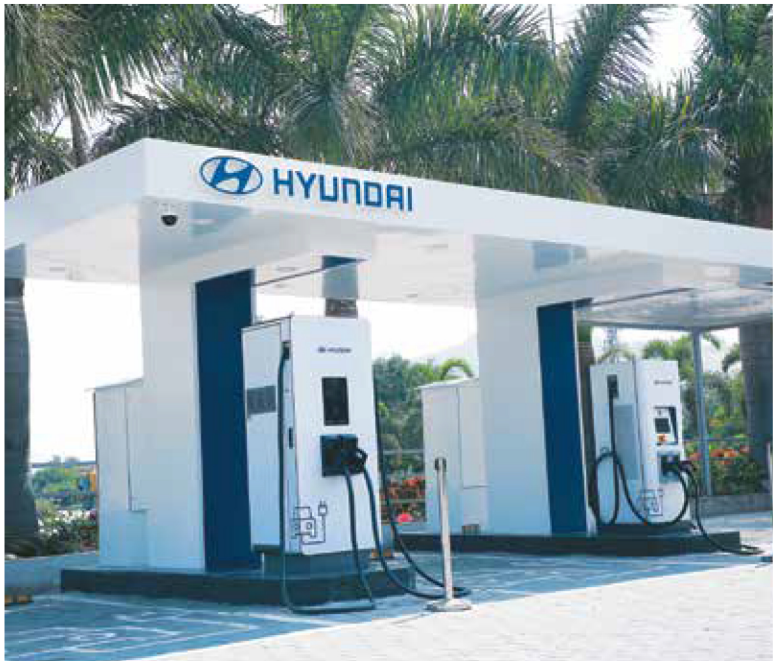
Hyundai DC charging station
